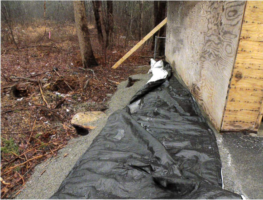
3. View of the south side of the garage with cut trees and crushed stone to be removed.
