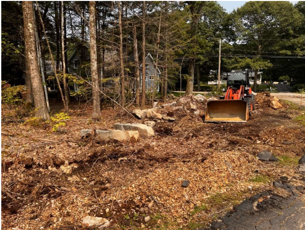
Photo 8 (07-17-23): Site clearing along north side of existing driveway facing Long John Road.
