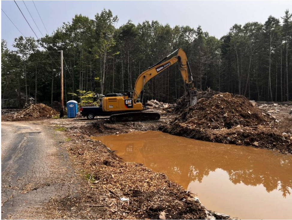
Photo 1 (07-17-23): Excavated area of drainage swale toward area of proposed driveway for single family unit.
