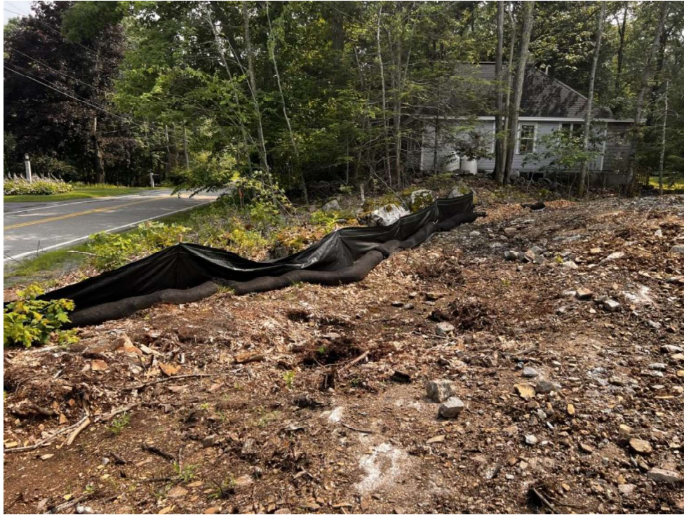
Photo 11 (07-17-23): Ledge removal taking place along the site entrance by use of hoe-ram.
