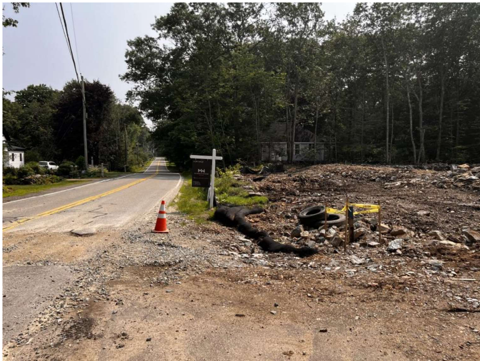
Photo 10 (07-17-23): Erosion control silt fence and silt sock installed on site along Long John Road.
