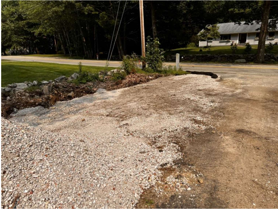
Photo 7 (07-17-23): North side of main entrance to site with erosion control silt sock placed at Long John Road.
