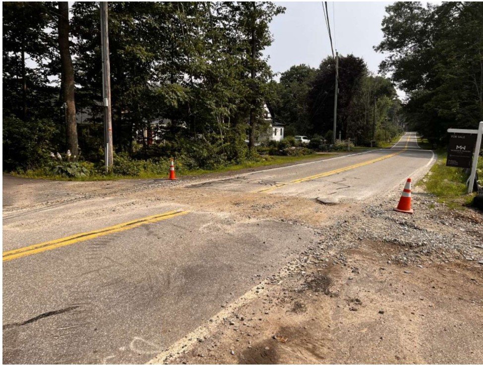
Photo 9 (07-17-23): Site entrance at Long John Road with trench cut for water main installation.
