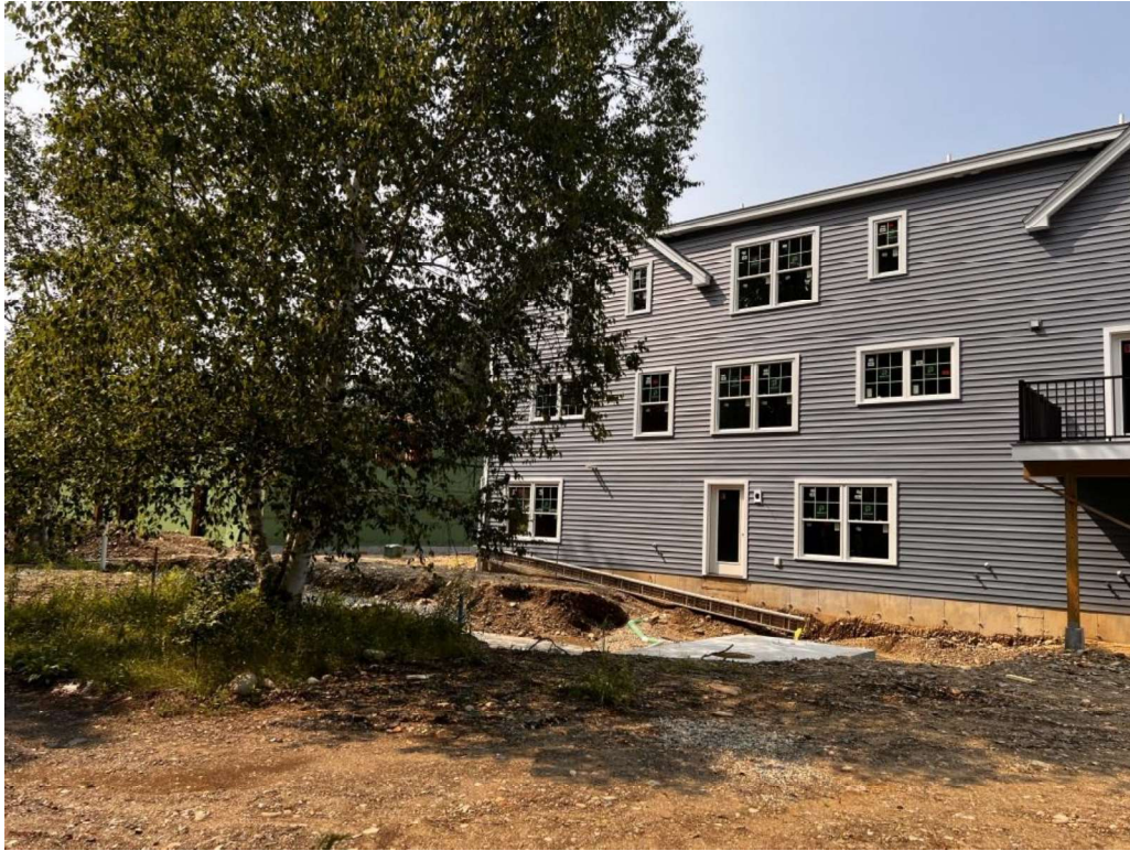
Photo 7 (07-17-23): Overall view of south side of site with constructed Building Units 28 to 30.
