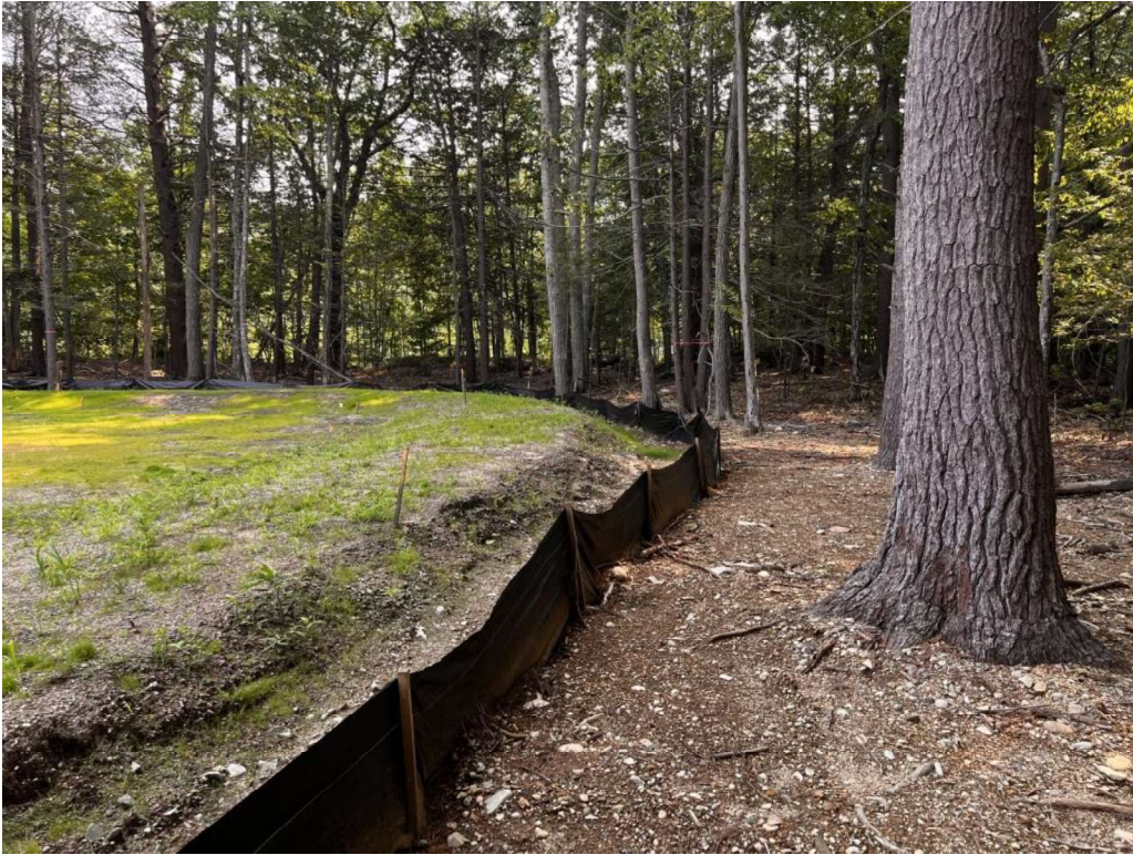
Photo 11 (07-17-23): Erosion control filter barrier has been reinstalled along the westerly property line behind the Grassed Infiltration Basin.
