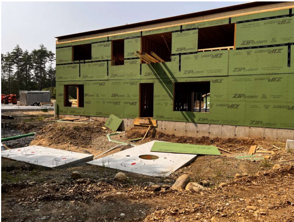
Photo 8 (07-17-23): Overall view of septic tanks installed to the south of Building Units 25 to 27.
