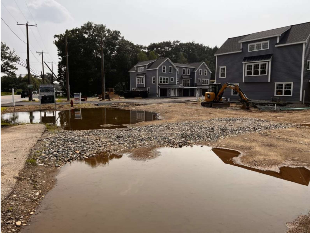
Photo 1 (07-17-23): Overall view of the northerly construction entrance to Lafayette Road. Stone will need to be touched up with stone and monitored during construction. Puddles are from recent rainstorm during the prolonged and ongoing rainy period.
