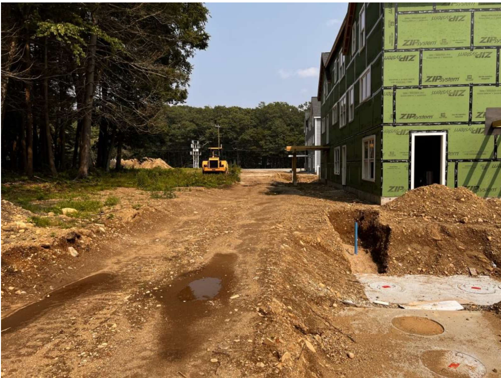
Photo 16 (07-17-23): Temporary construction access road along north side of site in good condition.
