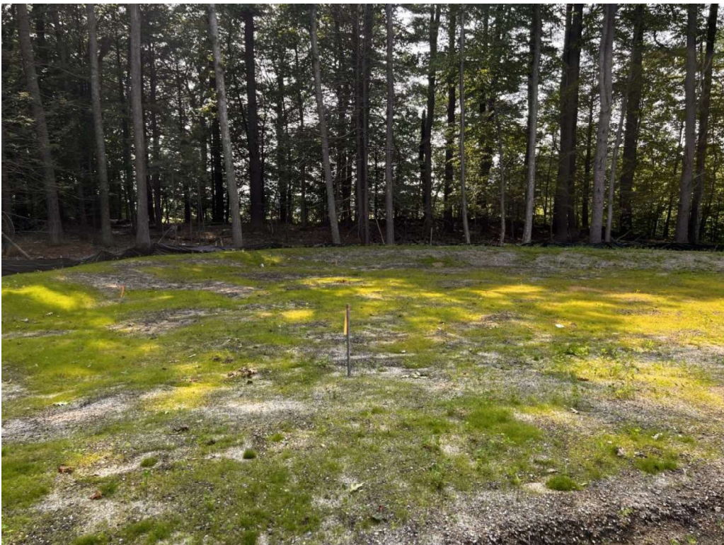
Photo 10 (07-17-23): Constructed infiltration basin sparse grassed area to be touched up.
