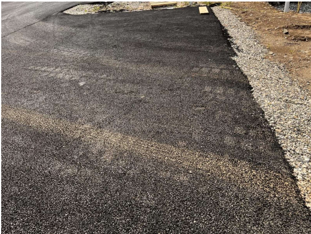
Photo 14 (07-17-23): Tracked sediment from site noted in various locations to be monitored and cleaned up as necessary.
