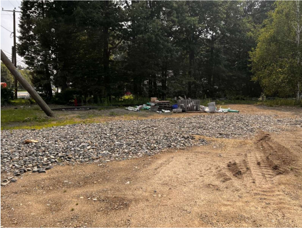
Photo 5 (07-17-23): Stabilized construction entrance placed at the south side of the site with no tracking on Lafayette Road.
