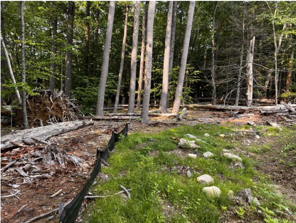
Photo 12 (07-17-23): Erosion control filter barrier to be installed around the north corner of property line behind the stockpile.
