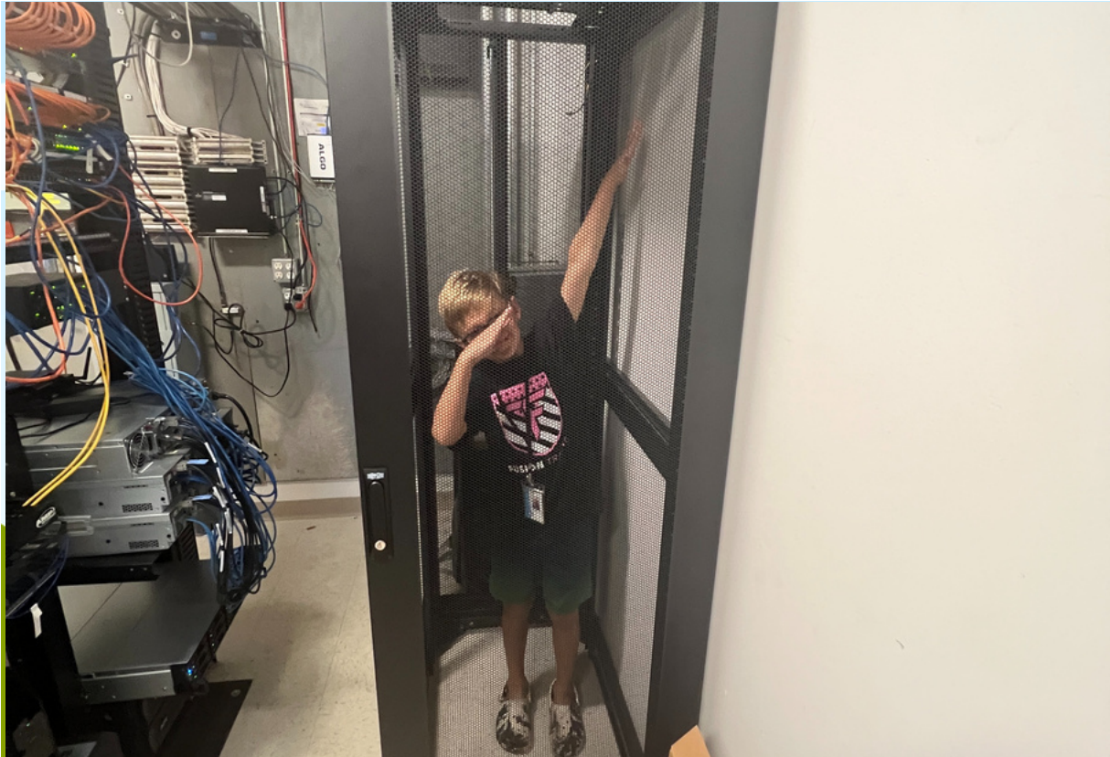
Early phases of Data Center Reconstruction. Bode for scale. On the left you can see the old servers, precariously perched on a shelf.
