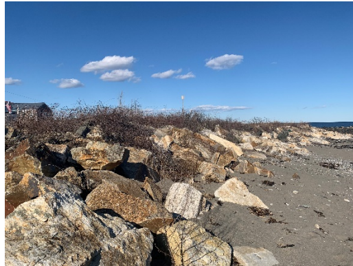
Loosely Placed Revetment Stone Facing Looking Northeast
