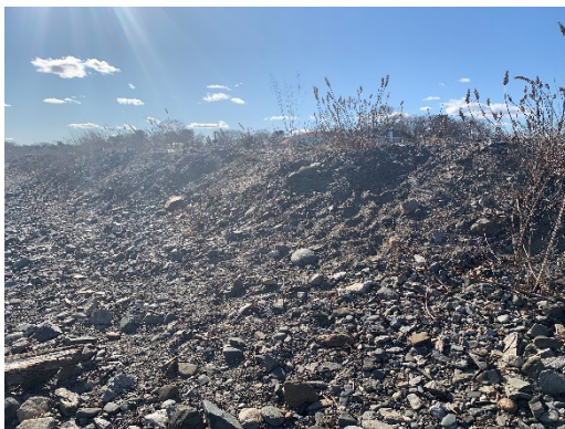
Shale Pile; Evidence of Erosion Looking West
