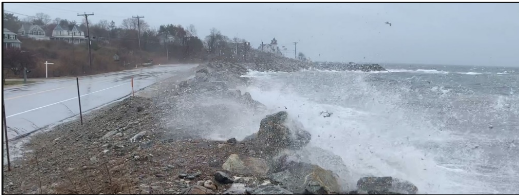
Photograph 1: Revetment Section 5 During April 9, 2020 Storm
