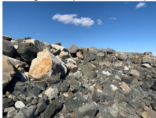
Revetment Stone Facing; Variable Size; Possible Subsidence - Looking Northeast ( \pm Sta. 783-End Sect.)
