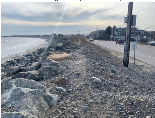
Top of Revetment; Loosely Placed Revetment Stone Looking Southwest (±Sta. 668)
