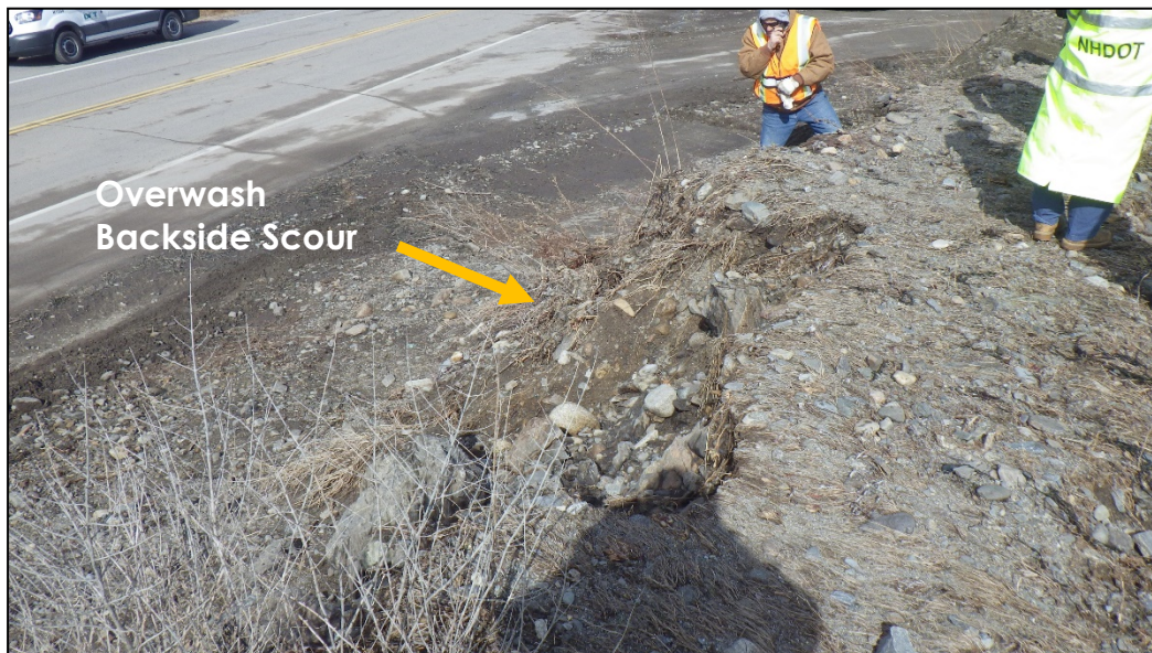
Photograph 3: Evidence of Shale Damage from Wave Overtopping After March 2018 Storms
