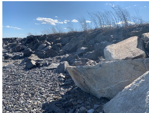
Loosely Placed Revetment Stone Facing Looking Southwest
