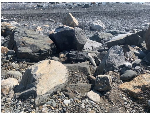
Revetment Stone; Evidence of Revetment Damage – Looking East (±Sta. 301+50)
