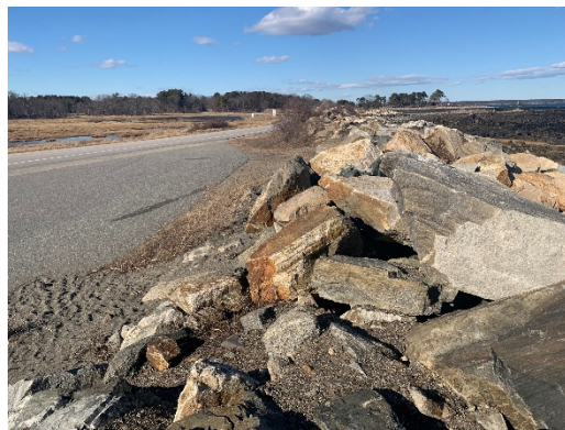
Top of Revetment; Voids Looking Northeast
