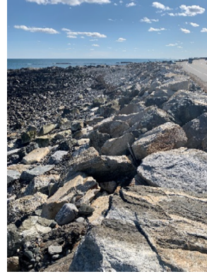
Top of Revetment; Voids Between Stone Looking Southeast
