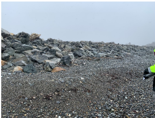
Revetment Stone; Evidence of Revetment Damage – Looking Northwest (±Begin Sect.)
