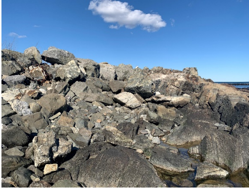
End Revetment/Beginning Bedrock Outcrop; Large Voids Evident - Looking Northeast ( \pm Sta 783+50)
