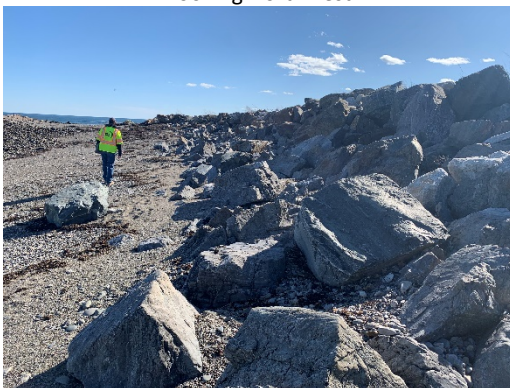
Shale Pile; Loosely Placed Revetment Stone Facing Looking Southeast (±Sta. 813)
