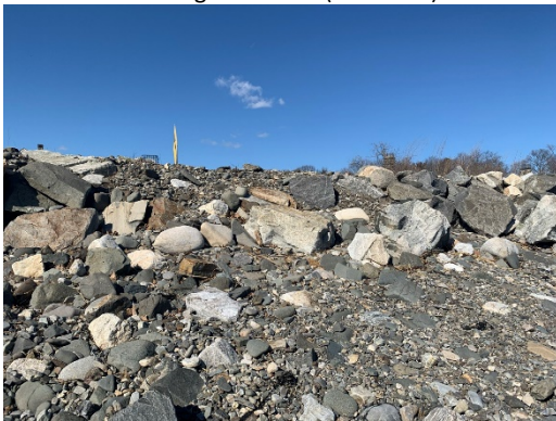
Shale Pile; Sporadic and Sparse Revetment Stone Looking West ( \pm Sta. 773 – Sta. 780+50)
