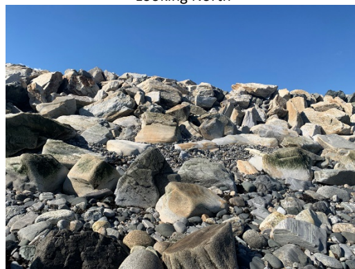
Loosely Placed Revetment Stone Facing; Possible Damage - Looking West (±Sta. 770)
