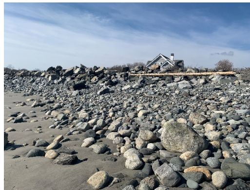
Loosely Placed revetment Stone Near Top of Slope Looking Southwest (±334+50)
