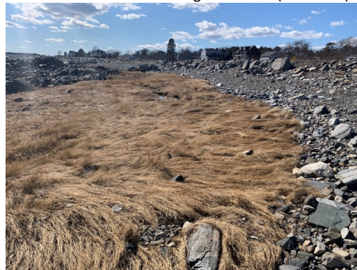
Shale Pile; Sporadic and Sparse Revetment Stone Looking Southwest ( \pm Sta. 773 – Sta. 780+50)
