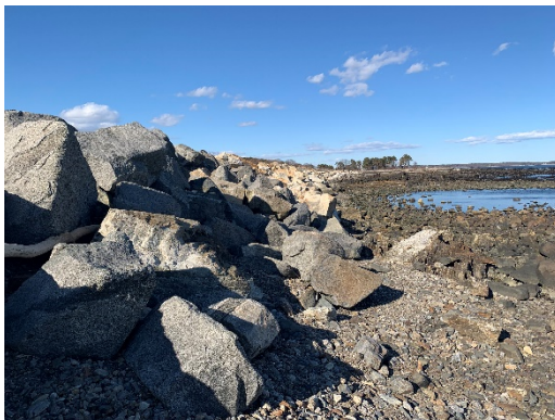
Revetment Stone Facing; Potential Displaced Stone Looking Northeast towards Section 1
