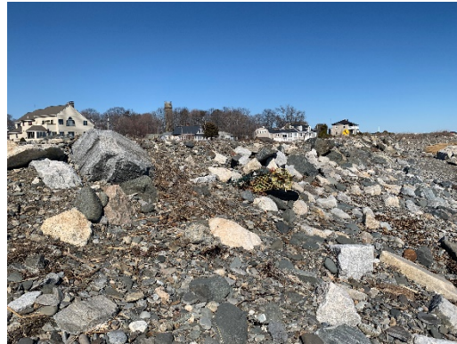
Begin Revetment/End Beach Access; Sparse Revetment Stone - Looking Northeast ( \pm Sta. 776)
