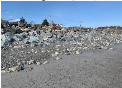
Loosely Placed Revetment Stone Looking North (±Sta. 664+10)
