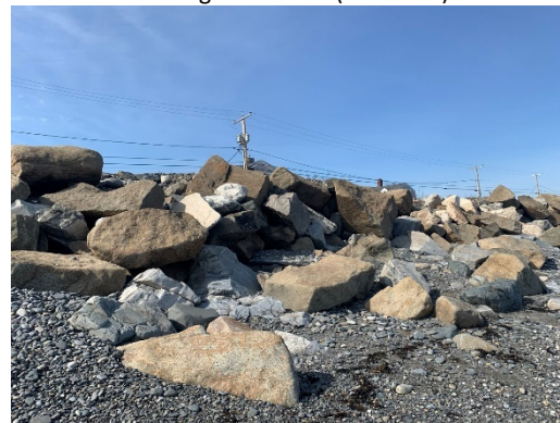
Loosely Placed Revetment Stone/Possible Damage Looking Northwest (±Sta. 641)
