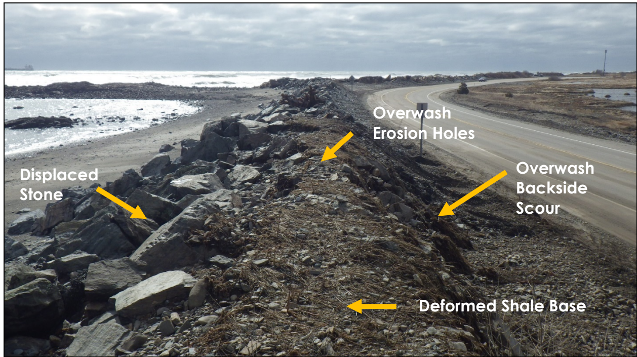
Photograph 2: Evidence of Revetment Damage After March 2018 Storms
