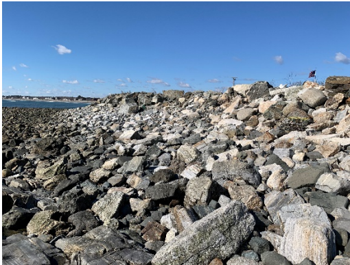
Loosely Placed Revetment Stone Facing Looking Southwest (±Sta. 683)
