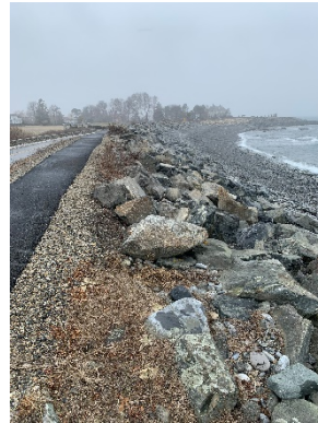
Top of Revetment; Possible Damage Looking North ( \pm Begin Sect.)
