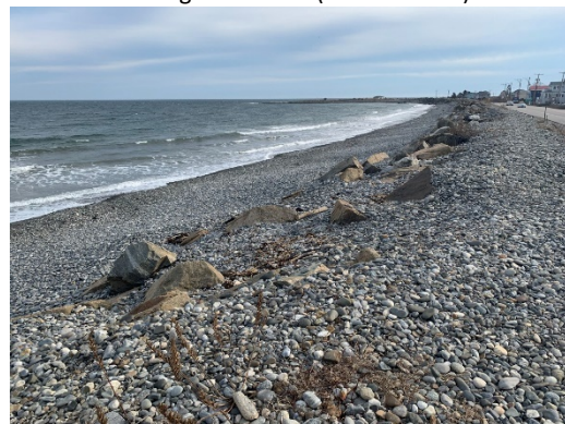
Top of Revetment; Sporadic and Sparse Revetment Stone - Looking South (±Sta. 650+50)
