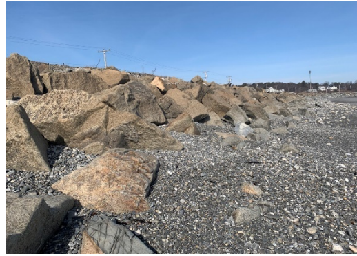
Loosely Placed Revetment Stone Looking North (±Sta. 659+30)
