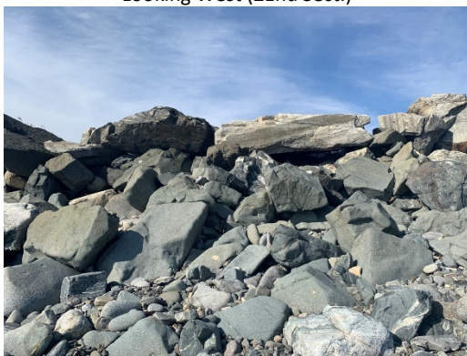
Loosely Placed Revetment Stone; Possible Revetment Damage - Looking West (±341+50)
