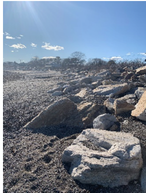
Loosely Placed Revetment Stone Facing Looking Southwest
