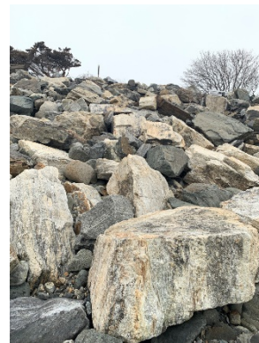
Revetment Stone; Evidence of Revetment Damage – Looking Northwest (±Begin Sect.)
