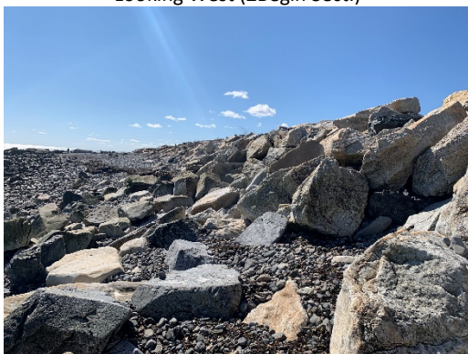
Revetment Stone Facing; Evidence of Subsidence Looking South
