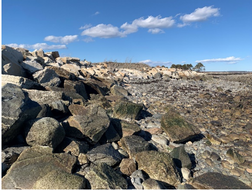
Shale Pile; Loosely Placed Revetment Stone Facing Looking Northeast (±Sta. 813)
