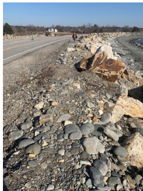
Revetment Stone; Evidence of Revetment Damage – Looking North (±Begin Sect.)
