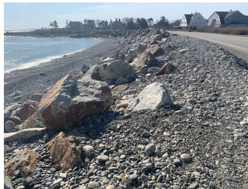
Revetment Stone; Evidence of Revetment Damage - Looking South (±Sta. 300+75)
