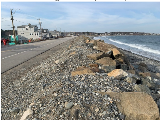
Top of Revetment; Loosely Placed Revetment Stone; Evidence of Revetment Subsidence - Looking North (±Sta. 639)
