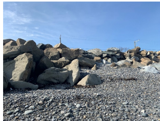
Loosely Placed Revetment Stone/Possible Damage Looking Northwest (±Sta. 637)
