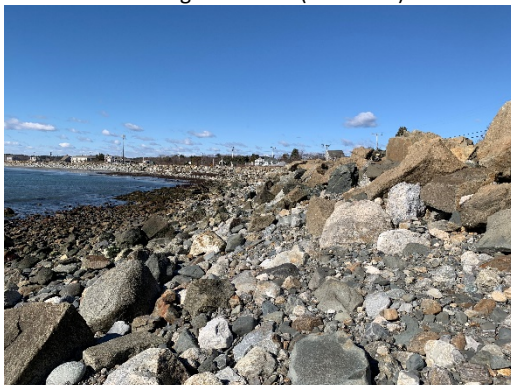
Loosely Place Revetment Stone Facing; Variable Stone Size/Gap in Revetment - Looking West (±Sta. 676+50)
