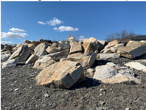
Shale Pile; Loosely Placed Revetment Stone Facing; Possible Damage - Looking West ( \pm Sta. 781 - 783)
