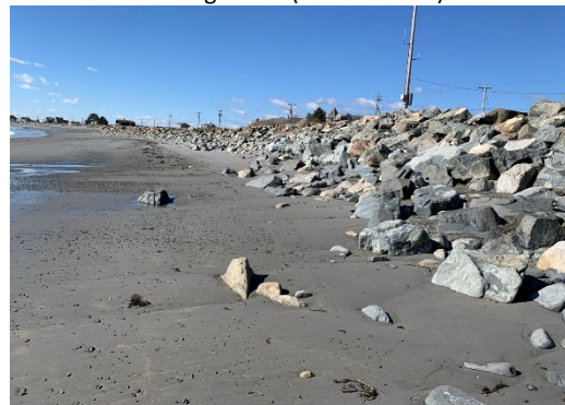
Loosely Placed Revetment Stone Looking Southwest (±Sta. 668+80)
