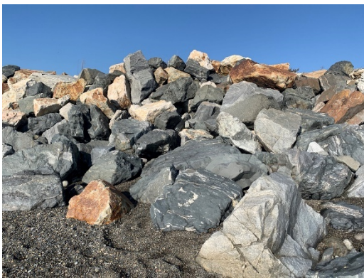
Revetment Stone; Possible Revetment Subsidence Looking Northwest (±Sta. 307)
