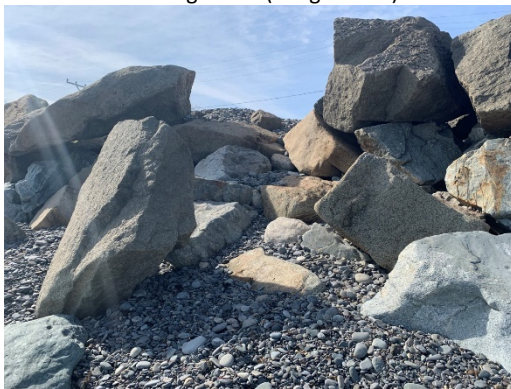
Erosion/Revetment Stone Subsidence Looking West (±Sta. 639+25)
