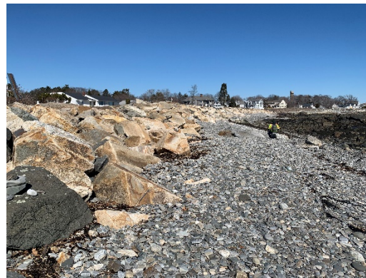
Loosely Placed Revetment Stone Facing Looking North
