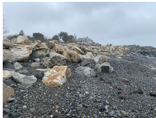
Loosely Placed Revetment Stone Looking North (±End Sect.)
