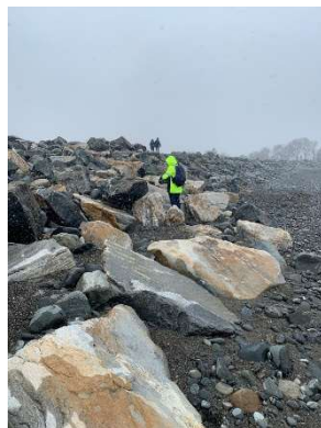
Revetment Stone; Evidence of Revetment Damage – Looking East (±Sta. 275)
