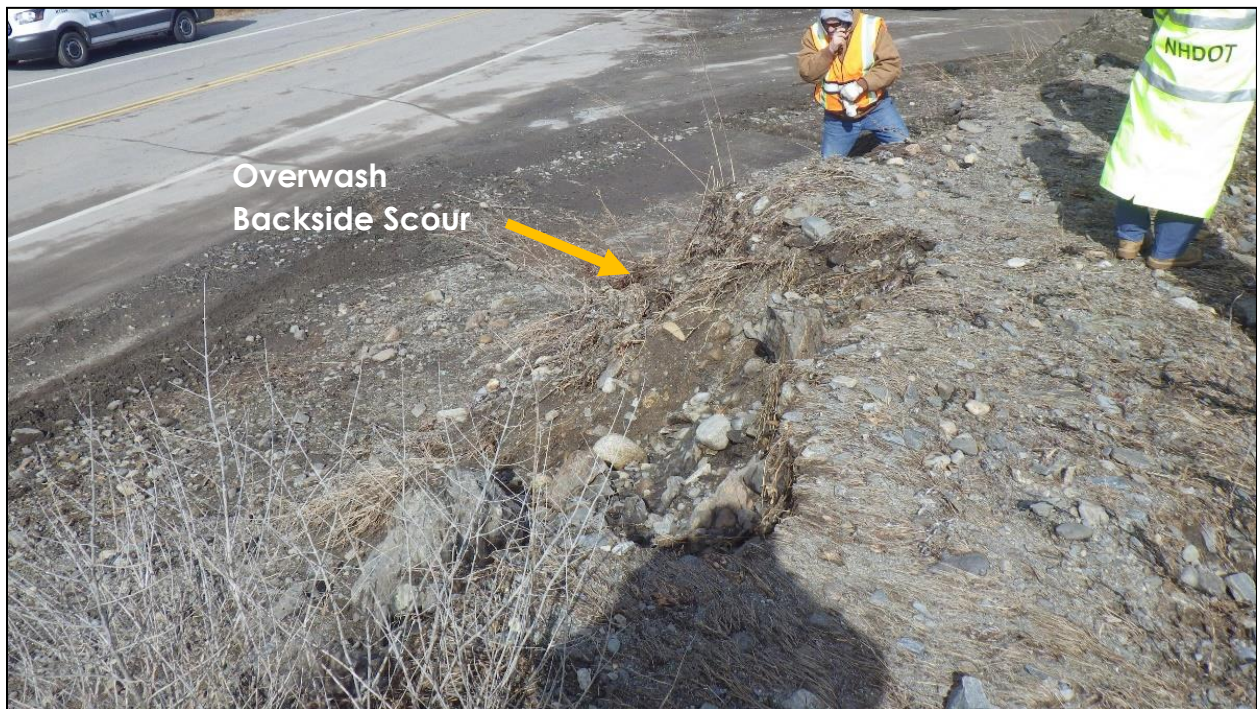
Figure 5: Evidence of Unprotected Shale Damage from Wave Overtopping After March 2018 Storms
