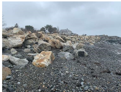
Loosely Placed Revetment Stone Looking North (±End Sect.)
