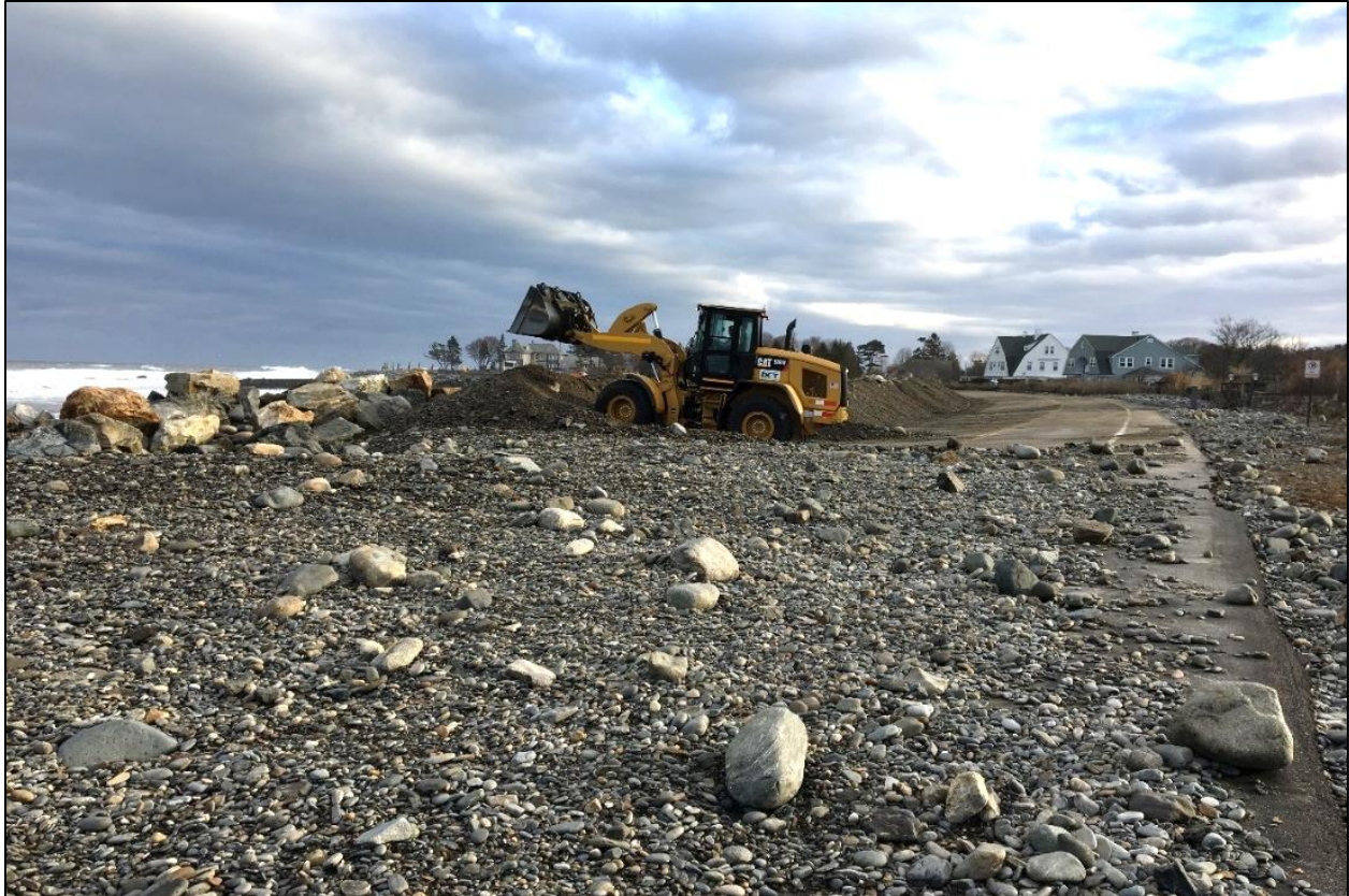
Figure 6: Stone Overwash Cleanup After March 2018 Storms
