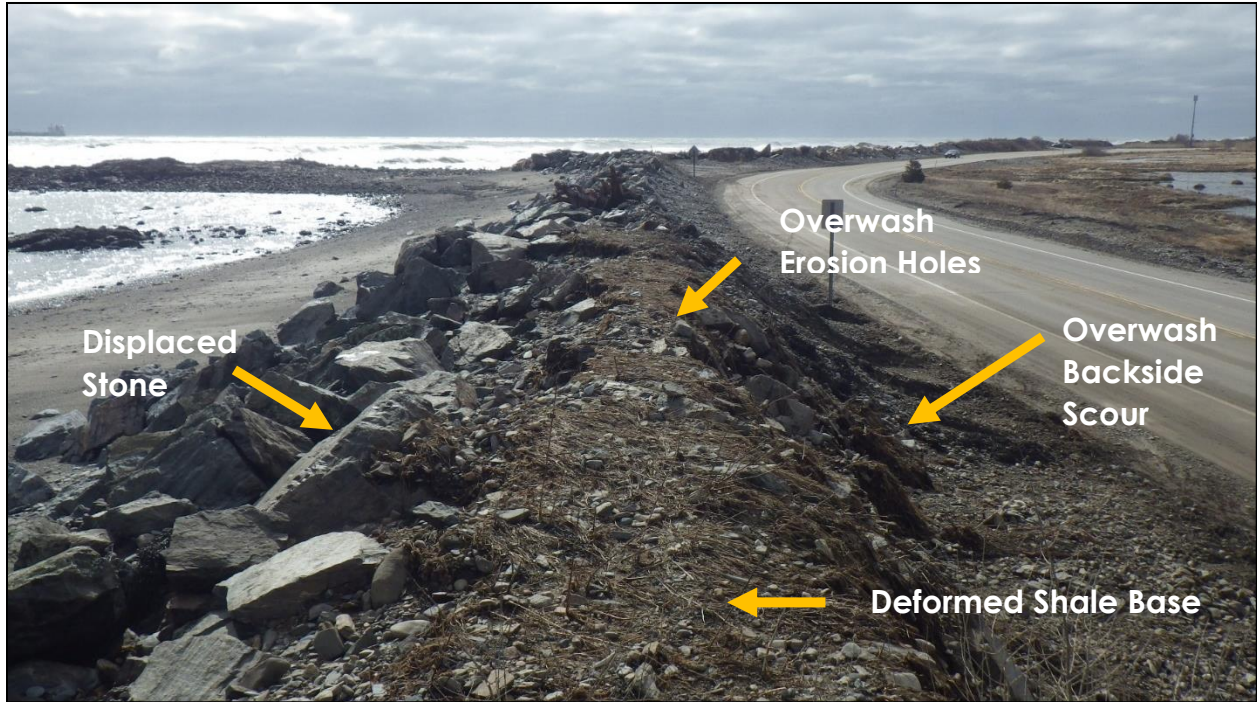
Figure 4: Evidence of Revetment Damage After March 2018 Storms
