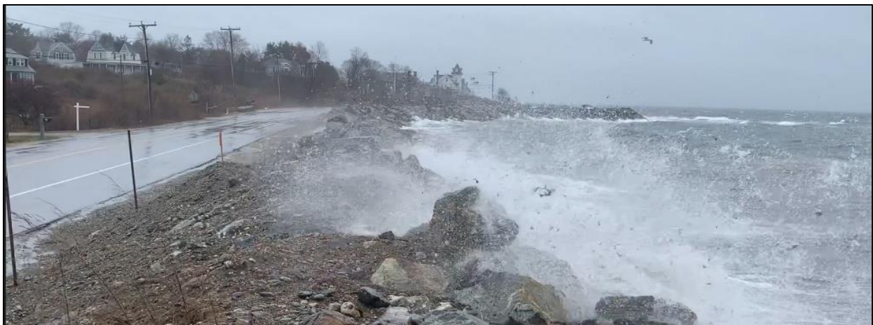
Figure 9: Revetment Section 5 During April 9, 2020 Storm
