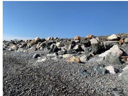
Revetment Stone; Evidence of Revetment Damage – Looking Southwest
