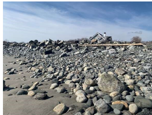
Loosely Placed revetment Stone Near Top of Slope Looking Southwest (±334+50)
