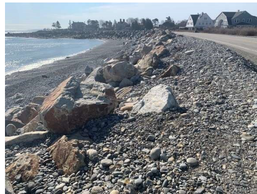
Revetment Stone; Evidence of Revetment Damage - Looking South (±Sta. 300+75)
