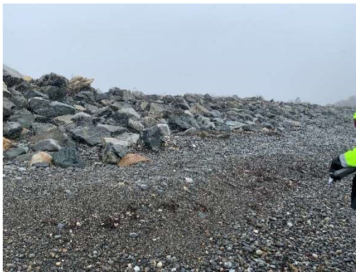
Revetment Stone; Evidence of Revetment Damage – Looking Northwest (±Begin Sect.)
