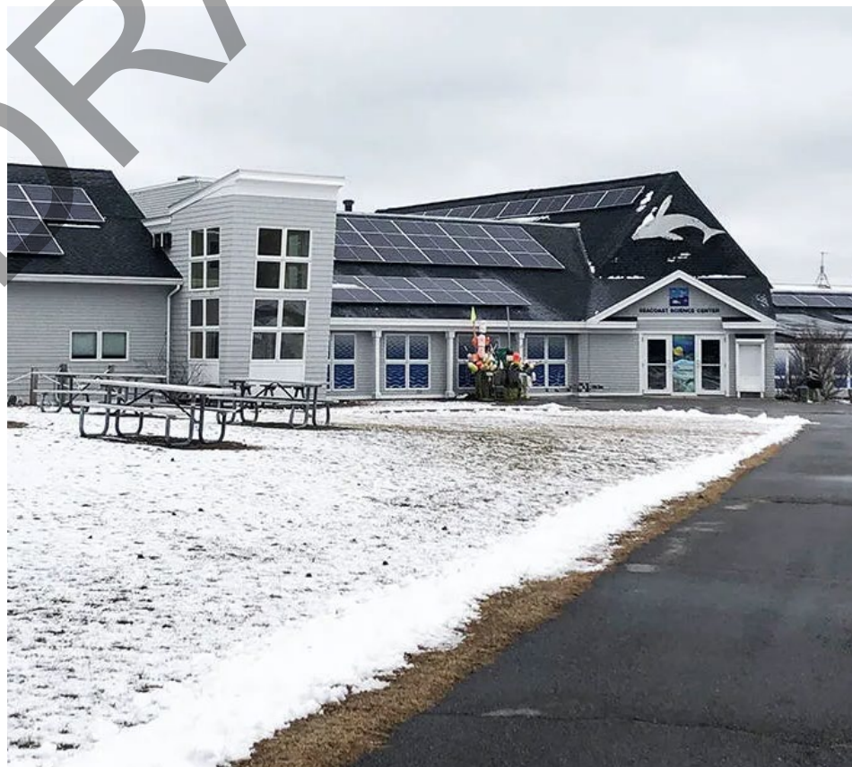
Above: Solar panels on the roof of the Seacoast Science Center in Rye, NH
